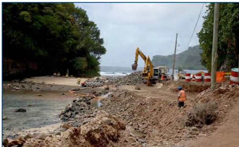
Photo 19: Road construction is an example of coastal development that can lead to anthropogenic stress on the territory's coral reef and shoreline resources.
