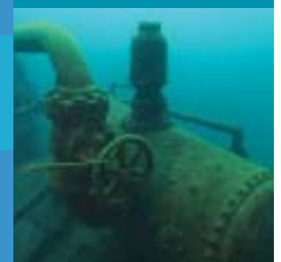
Boiler on the Thew . Photo: John Brooks
