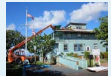
In addition to basic O&M costs, periodic overhauls and repairs are needed on facilities. The restoration work on this historic structure in Kīhei, Maui, will repair long term structural damage. Photo: Paul Wong
